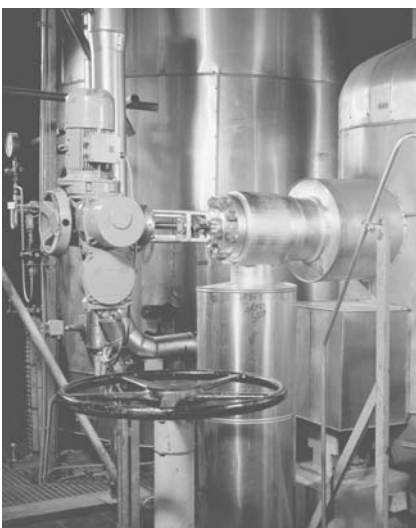
H.P. preheater in a nuclear power station equipped with a condensate drain control valve type ZK 29
