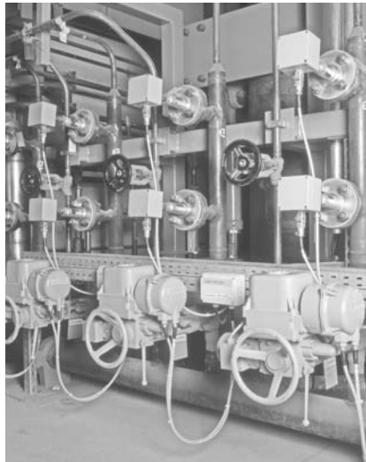
Drain control station using ZK 29 valves with electrical actuator
